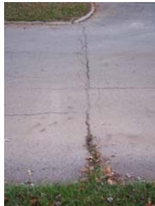
Example of high severity transverse reflective cracking on composite pavement
