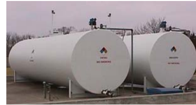
West 40 fuel tanks
