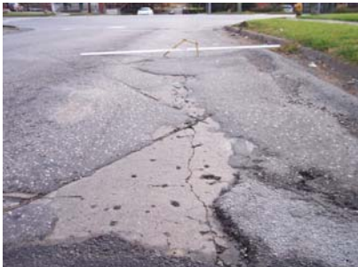
Example of high severity rutting and shoving on a composite pavement
