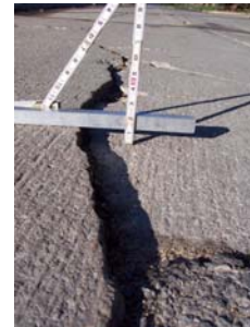
Example of a high severity fault failure in a rigid pavement
