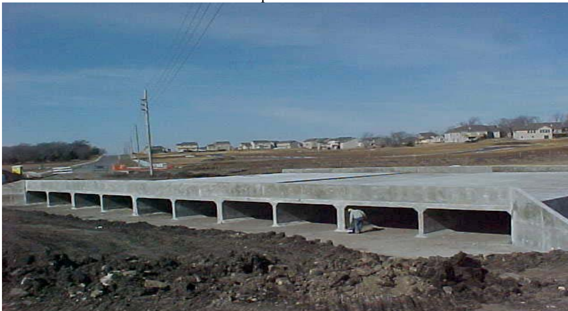
A multi-cell reinforced concrete box located on the Crossgate project is being inspected.
