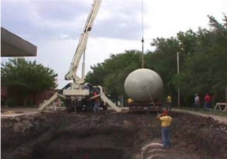
Crews lower a new fuel tank into the ground at 1140 Haskell Avenue.
