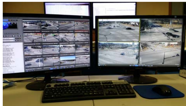
ITS Center (Intelligent Transportation System)
