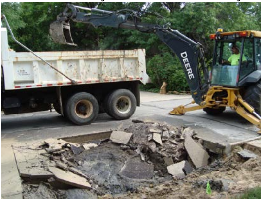
Crescent Road Sinkhole
