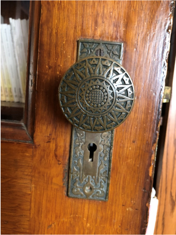
Figure 11: Original door hardware
