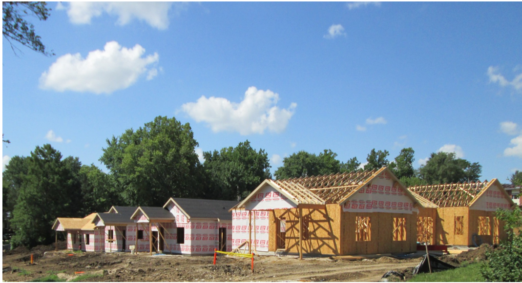
August 2015 photo of cottages being framed and insulated on the west side of 2500 Cedarwood, behind the United Way Center.
