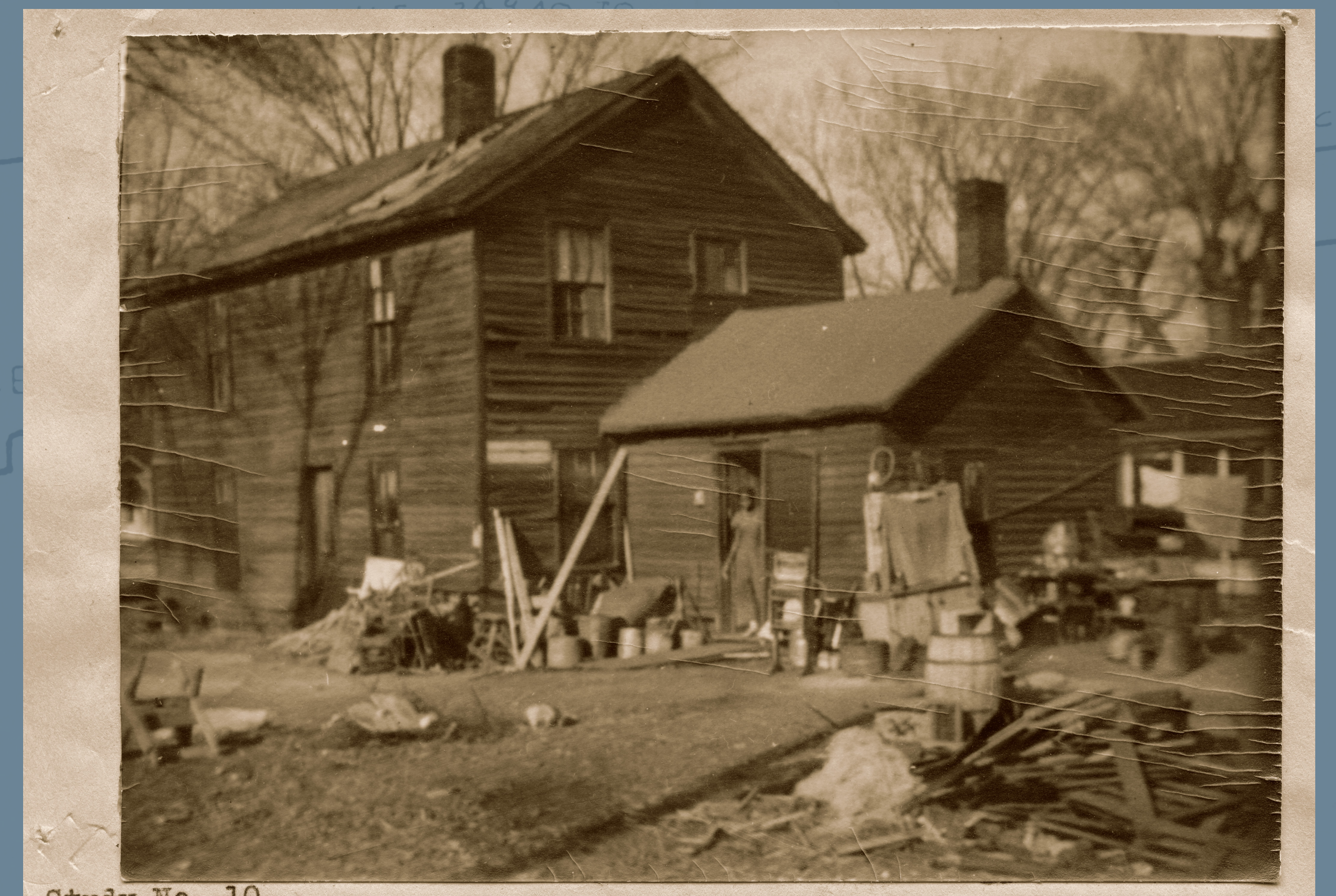
Study No. 10. Two families occupy this old derelict. Built as near as I could learn, in 1868. The upstairs is partly unused because the roof leaks into one room, and "The children might fall through the holes"
