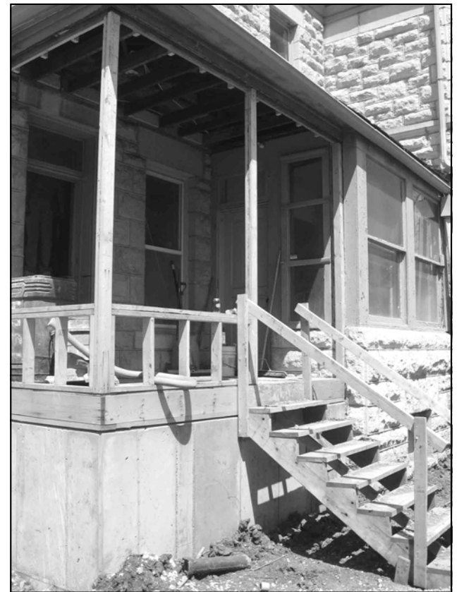
Fresh concrete and new stairs have refreshed the back porch where Libby spent many hours watching the Oread neighborhood go by.
