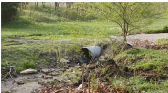
Figure 6. Newer culverted drive across the creek on the west side of the school property.
