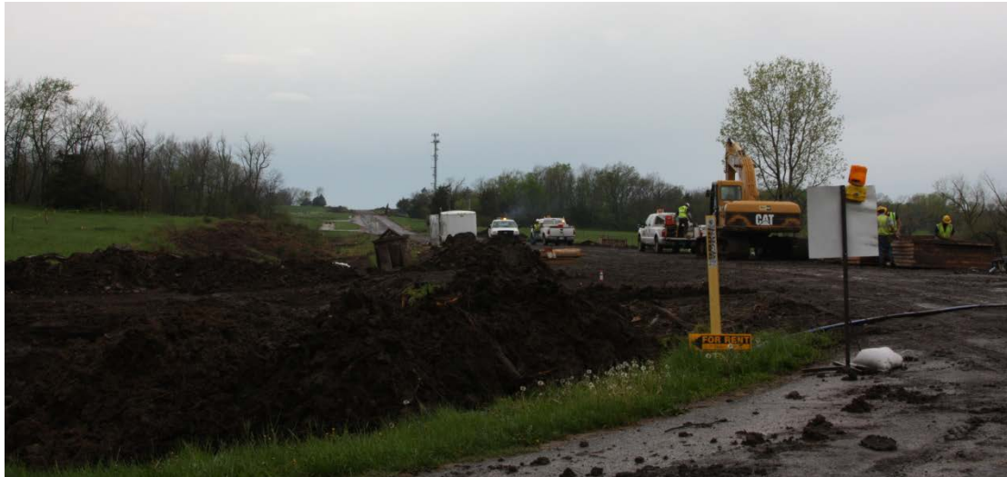
Figure 41. KDOT in the process of widening the middle box culvert on US Highway 56 at 11th Street. According to the inspector on-site, the cross section here (near 11th Street) will also include a 5 foot sidewalk on each side of the highway.
