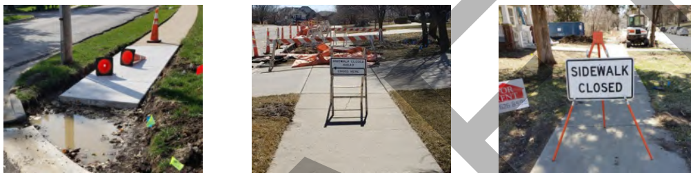
Figure B11: Incorrect Pedestrian Accommodations in Work Zones
