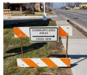
Early warning sign placed to the side of the sidewalk (where it is safe to cross) to allow access to local businesses
