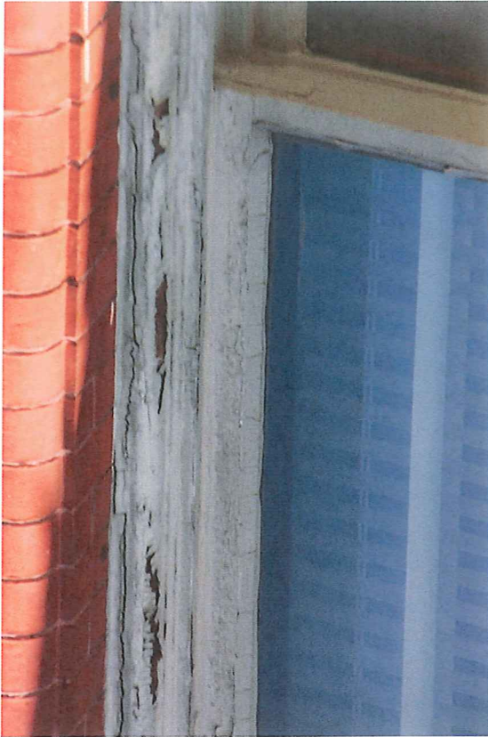
Window Detail: deteriorated paint
