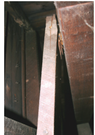
2x6 Hanger Supporting Ledger is Skewed 16"
