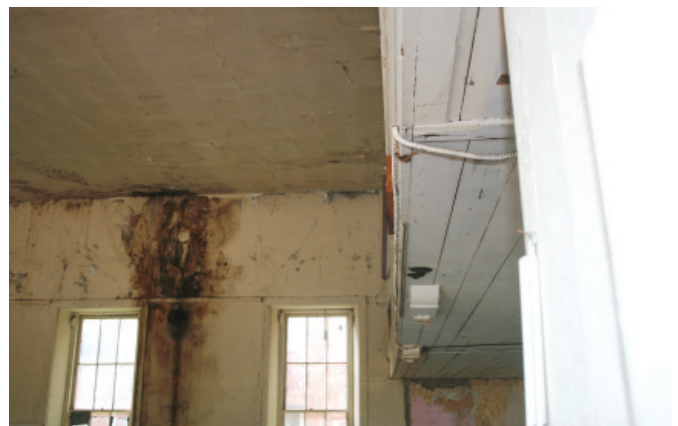
Bowing Balcony Framing
