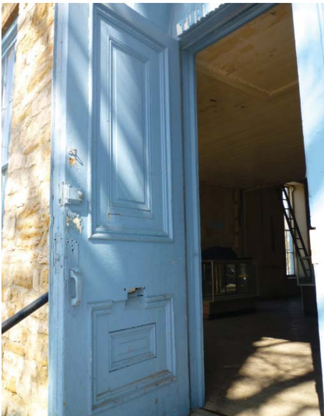
The main entrance doors exhibit moderate integrity. There have been several alterations made to the doors over the years, but these changes may be reversed and the doors restored.
