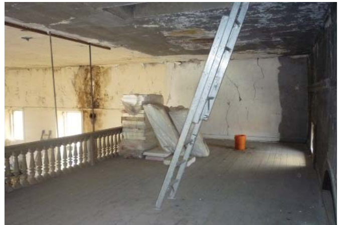
The architectural features of the balcony, including the wood balustrades, plasterwork and wood floor are significant features that should be retained and restored. Further investigations should be made into the decorative frieze on the west wall.
