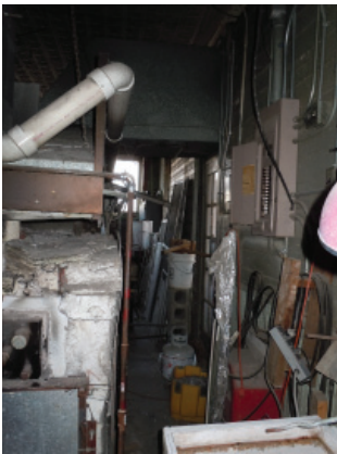
Main Electrical Power Panel
