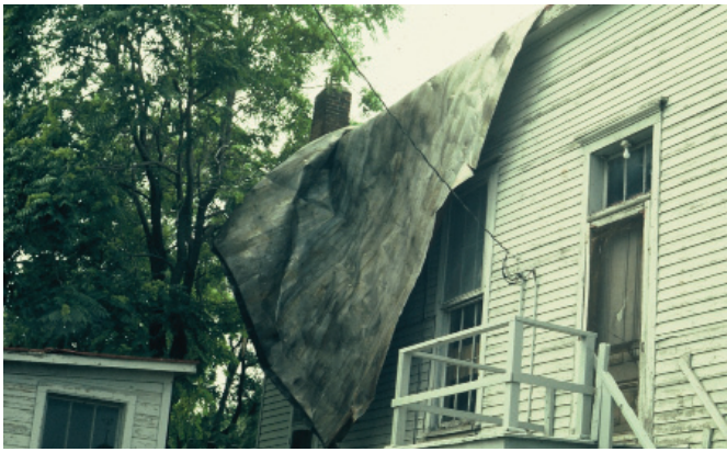
Storm Damage of Metal Roof, 1973 (Courtesy of Larry Miller). The storm damage photographs indicate a metal roofs at both the flat and gabled roofs prior to 1973.
