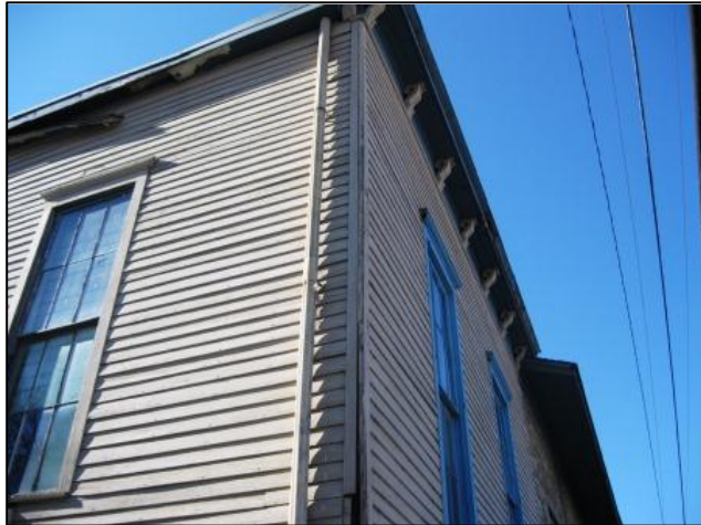
Deteriorated LBP on the exterior siding, trim, window, gutter/downspout components
