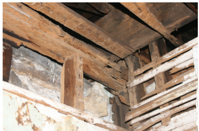
Badly Deteriorating Wood Bearing Wall at South End of Stage
