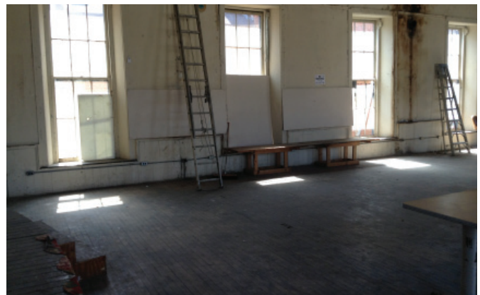
Surface Mounted Convenience Receptacles in 1st Floor Auditorium
