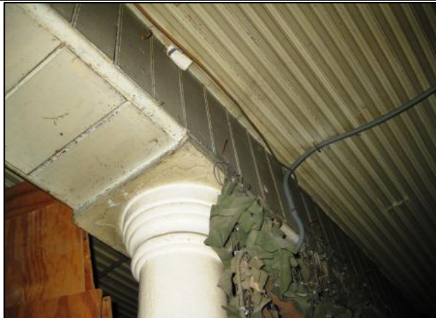
Deteriorated LBP on the interior basement ceiling, beam and column
