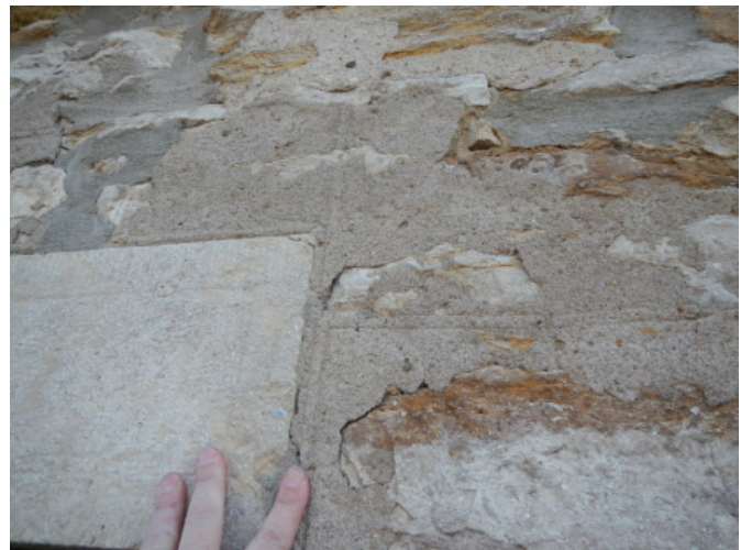
Evidence of Stucco Layer
