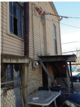
Main Overhead Electrical Service
