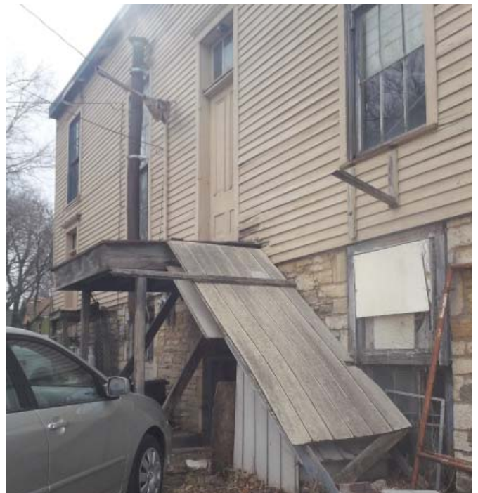
There are several features on the east elevation that exhibit low integrity. The rear wood stoops and steps are deteriorated and it is unclear how the exits have been modified over time. The windows on this elevation have also been modified by the insertion of exhaust ductwork. Enough material remains, however, to restore or replicate these features.
