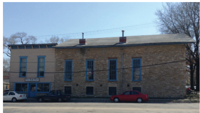
Gutter and Downspout for the North Roof Edge – Downspout is Disconnected from the Gutter
