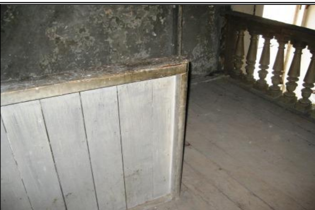
Deteriorated LBP on the interior balcony half wall, railing components, baseboards and floor
