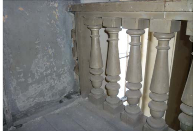
The original balustrade at the balcony level has high integrity as it is in excellent condition and has had no alterations.
