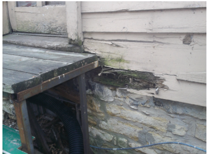
Deteriorated Wood Siding on East Elevation
