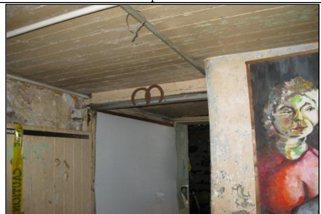
Deteriorated LBP on the interior basement bathroom walls and trim
