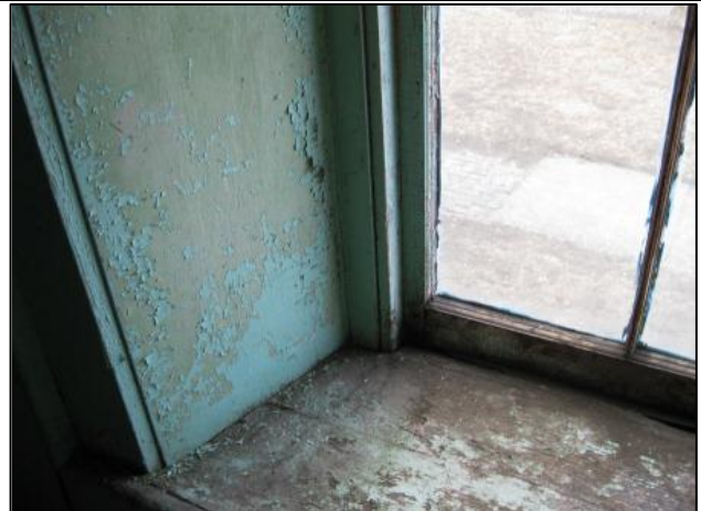
Deteriorated LBP on interior 1 st floor window components
