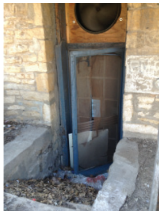
Exhaust Fan for Basement Ventilation Hood – Located Above the East Exit Door
