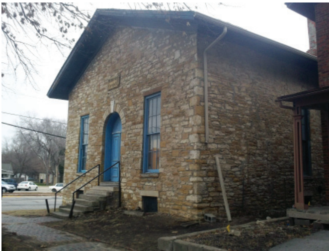
Disconnected Downspout at Southwest Corner (since reconnected)
