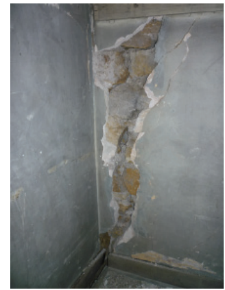
Plaster Deterioration as a Result of Structural Settlement
