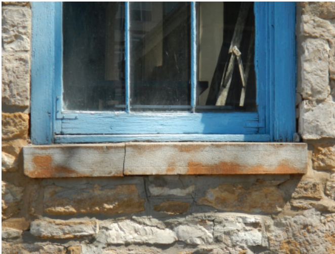
Cracked Window Lintel and Windowsill
