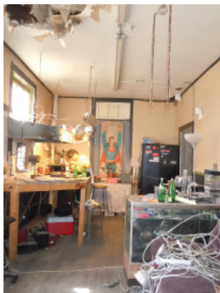
Lighting in 1st Floor Office
