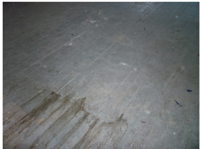
Stage Wood Floor. Scars in the stage floor and basement tin ceiling below indicate a change in configuration at the stage floor.
