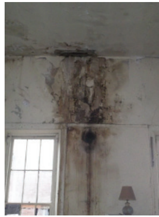
Water Damage at Flat Plasterwork
