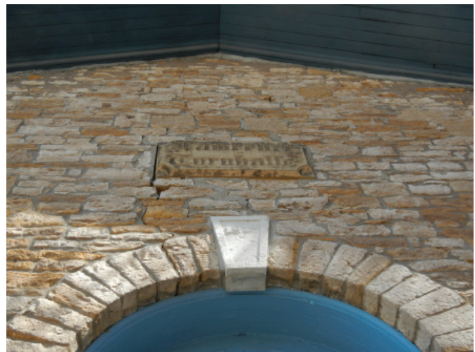
Vertical Crack Along Keystone and Cartouche on West Elevation
