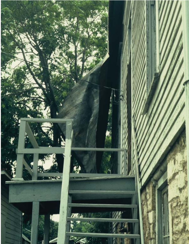
Storm Damage of Metal Roof, 1973 (Courtesy of Larry Miller).
