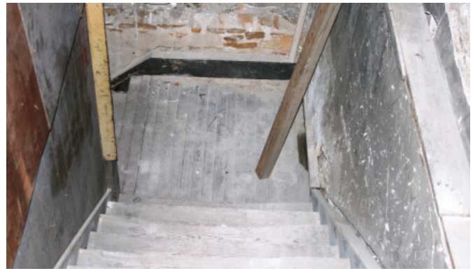
Unsupported Northwest Stair Landing
