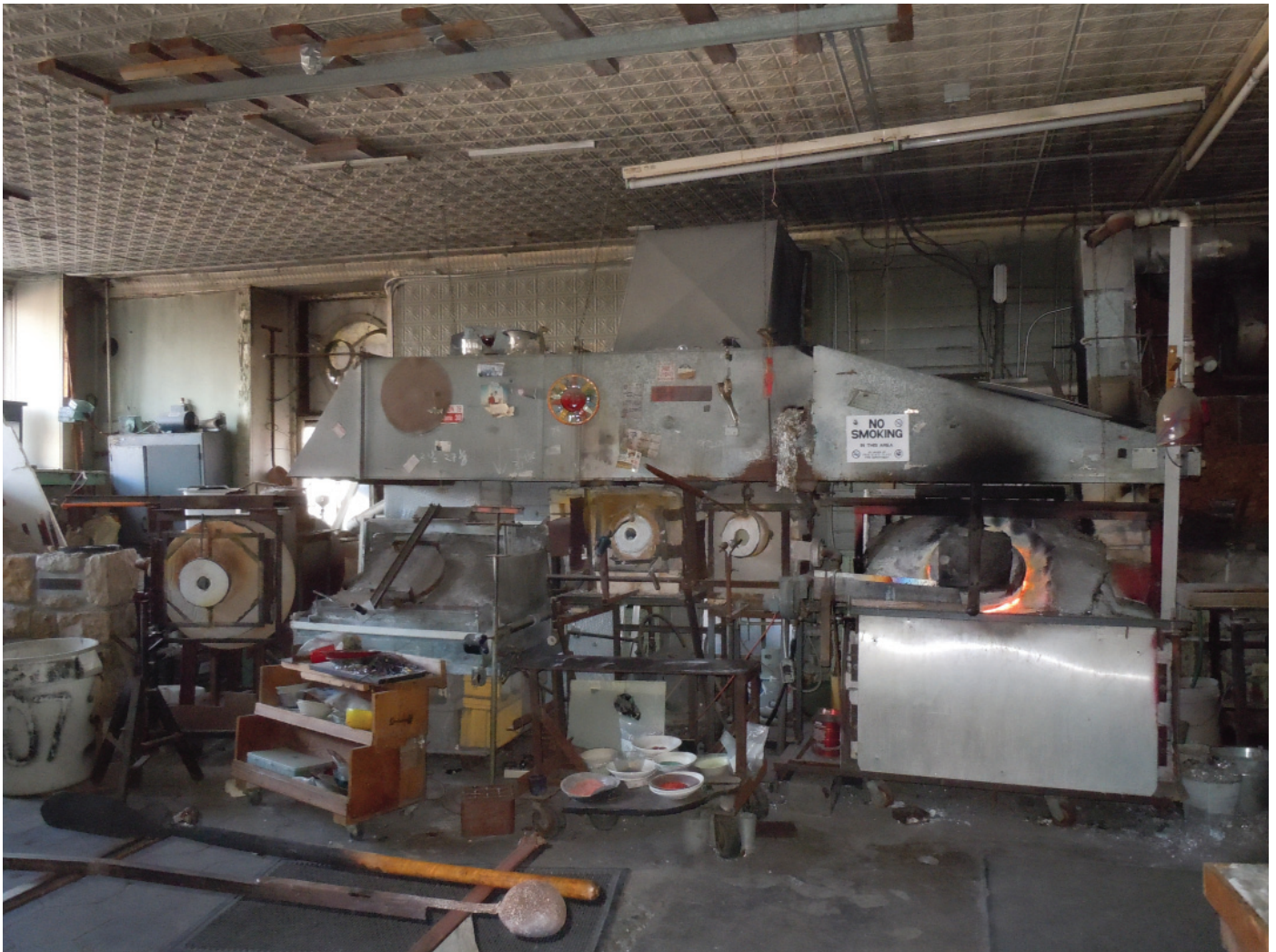
Basement Ventilation Hood
