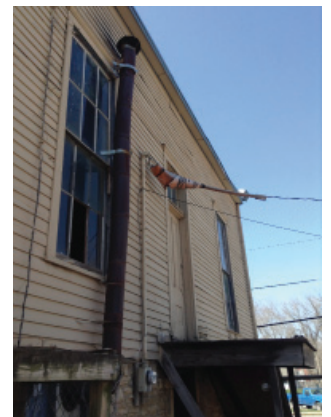
Flue for Glass Kilns – Located on Exterior of East Wall of Building
