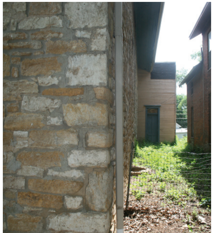
West Limestone Exterior Walls Bowing
