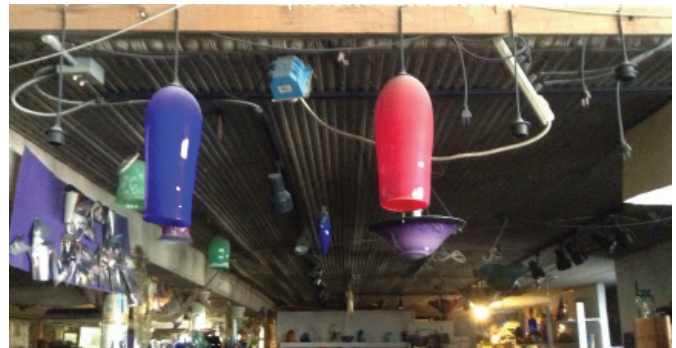
Lighting in Basement
