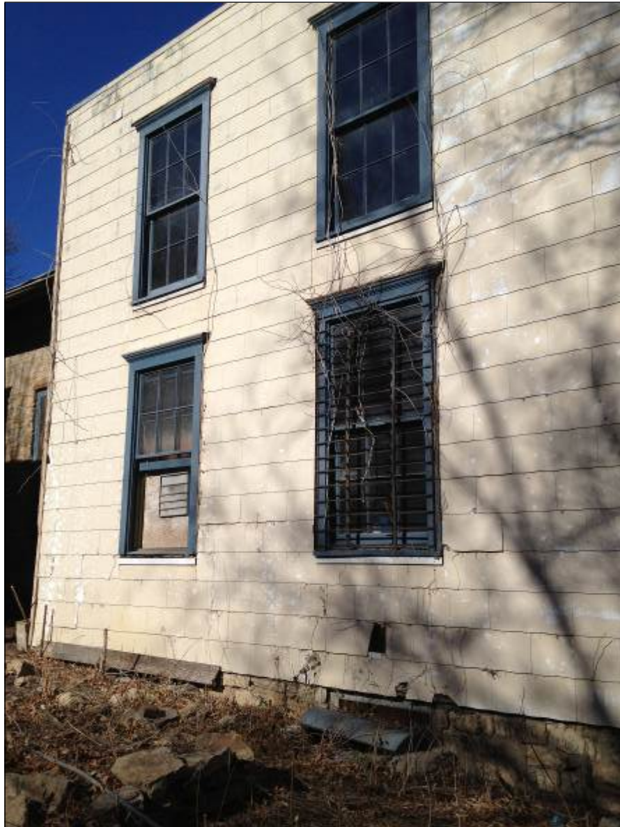
Asbestos containing siding on south rear side of building
