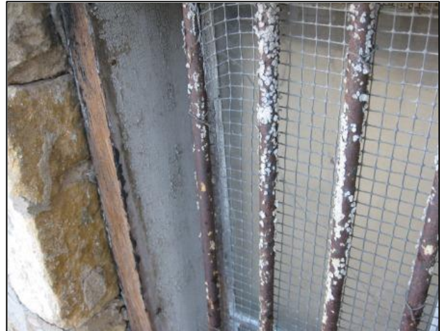
Deteriorated LBP on the exterior window components & window bars
