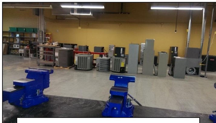
The Belcher Family HVAC Lab, December 2016
