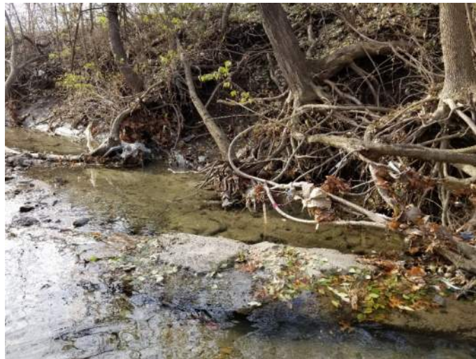
Figure 5 – Photo Looking Downstream at West Bank, Railing in Upper Left Corner of Image
