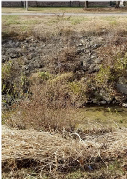
Figure 3 – Photo of Proposed Location of Perpendicular Crossing of Naismith Creek, Looking West from Dillon’s Parking Lot
