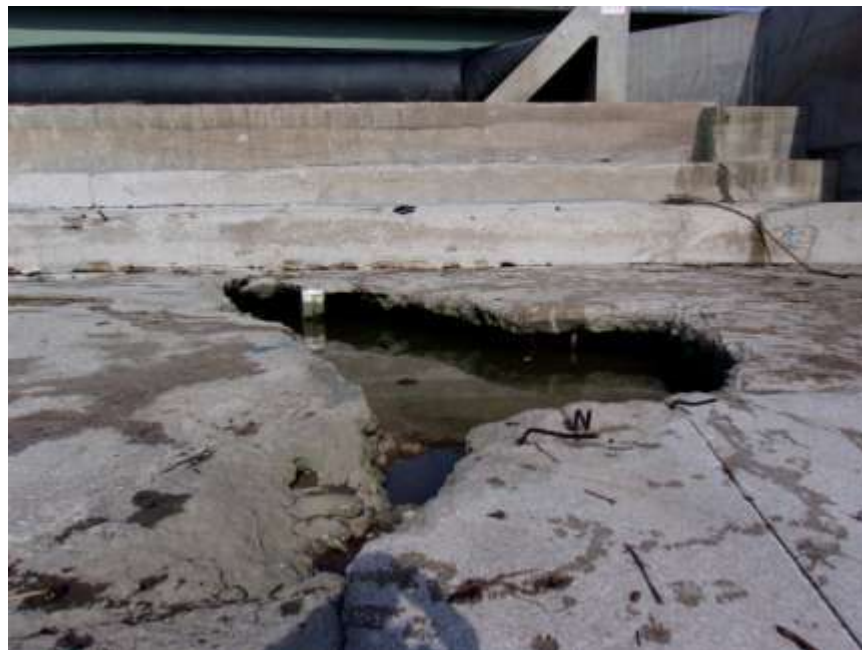
Dam Apron Scour Hole
