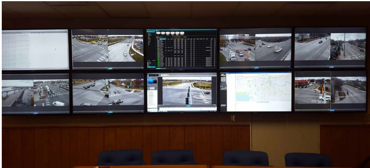
Traffic Operations Center
