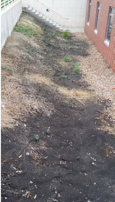
Drainage problem at Fire Station 5
