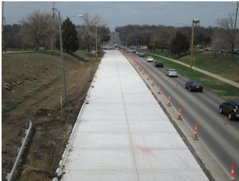
Iowa St. looking north from Irving Hill Road Bridge Southbound lanes complete
