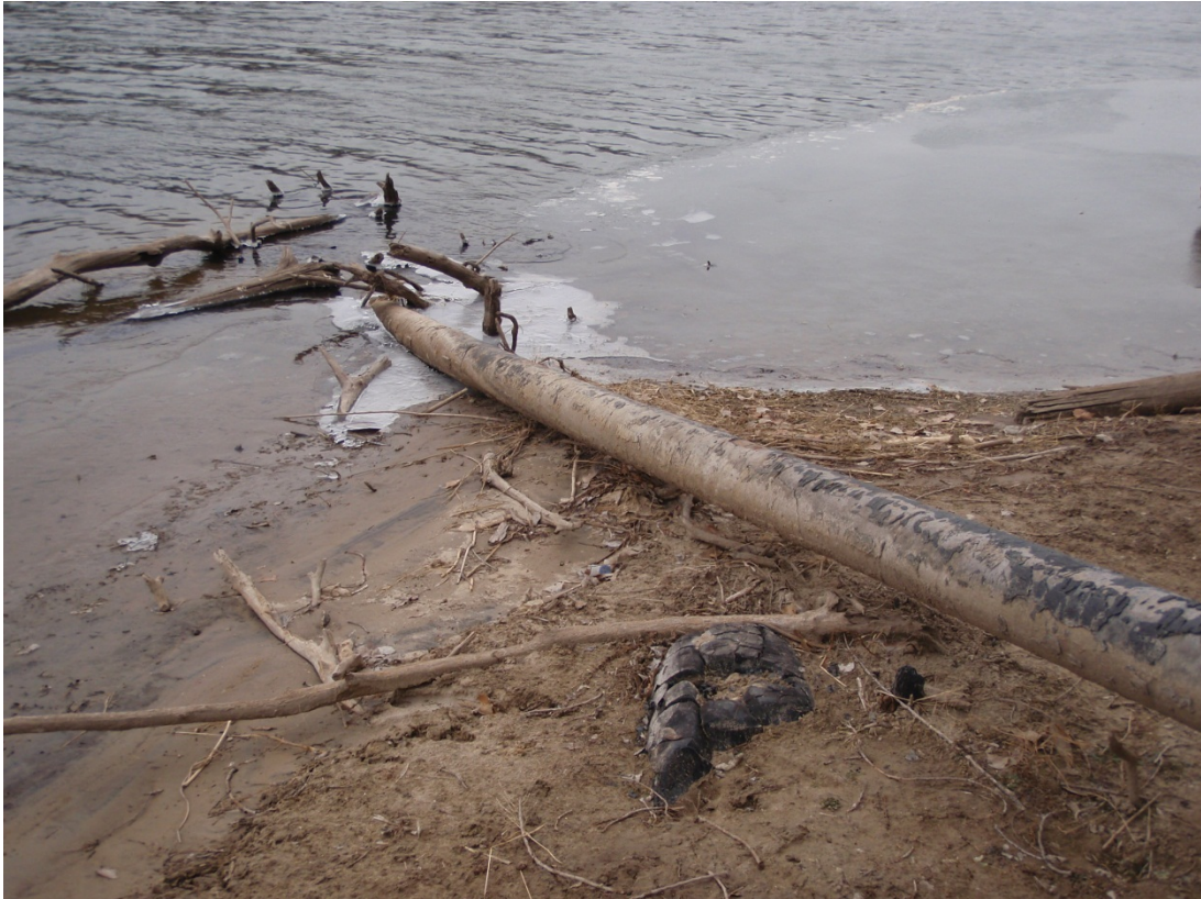
Exposed forcemain at water's edge.
