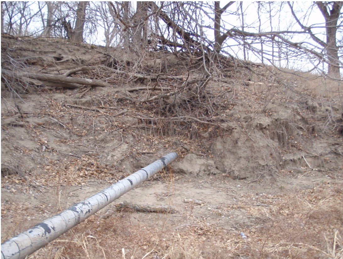
Exposed forcemain at nort bank.
