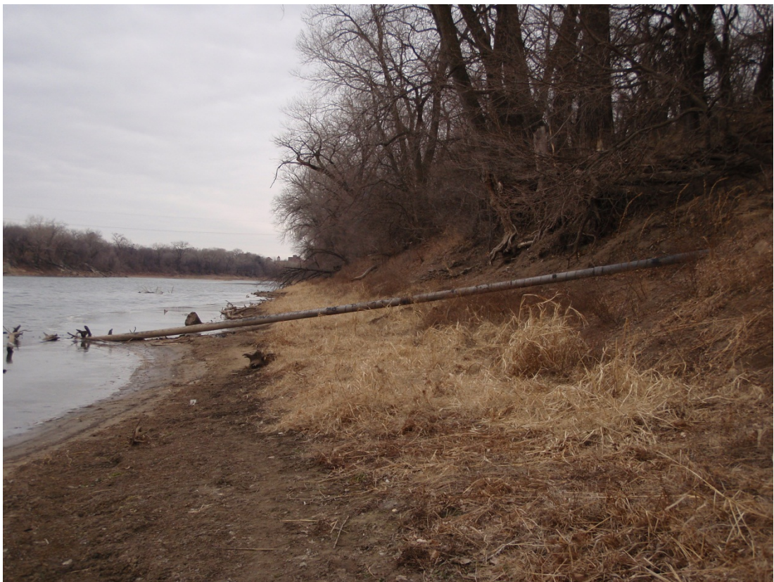
Exposed forcemain looking upstream.
