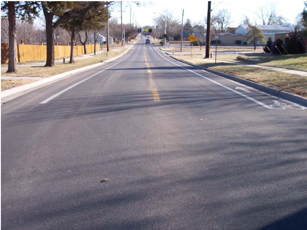
Description - Contracted Milling and Overlay w/ Pavement Markings & Bicycle Lanes on E 19 th St from Barker Ave to Almira Ave (E of Haskell Ave) as part of Emergency Rehabilitation
