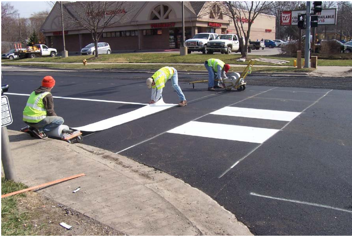
Description – Louisiana St near 23 rd St during Contracted Milling and Overlay Patching w/ Pavement Markings as part of Emergency Repair and Rehabilitation
