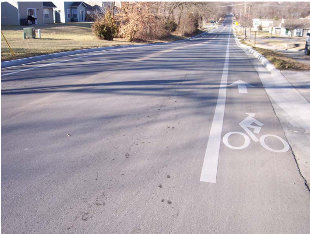
Description – Completed Overlay, Curb & Gutter Removal & Replacement, & w/ Bicycle Lane Pavement Markings on E 15 th St from Connecticut St to Haskell Ave as part of Contracted Milling & Overlay (Phase 2)
