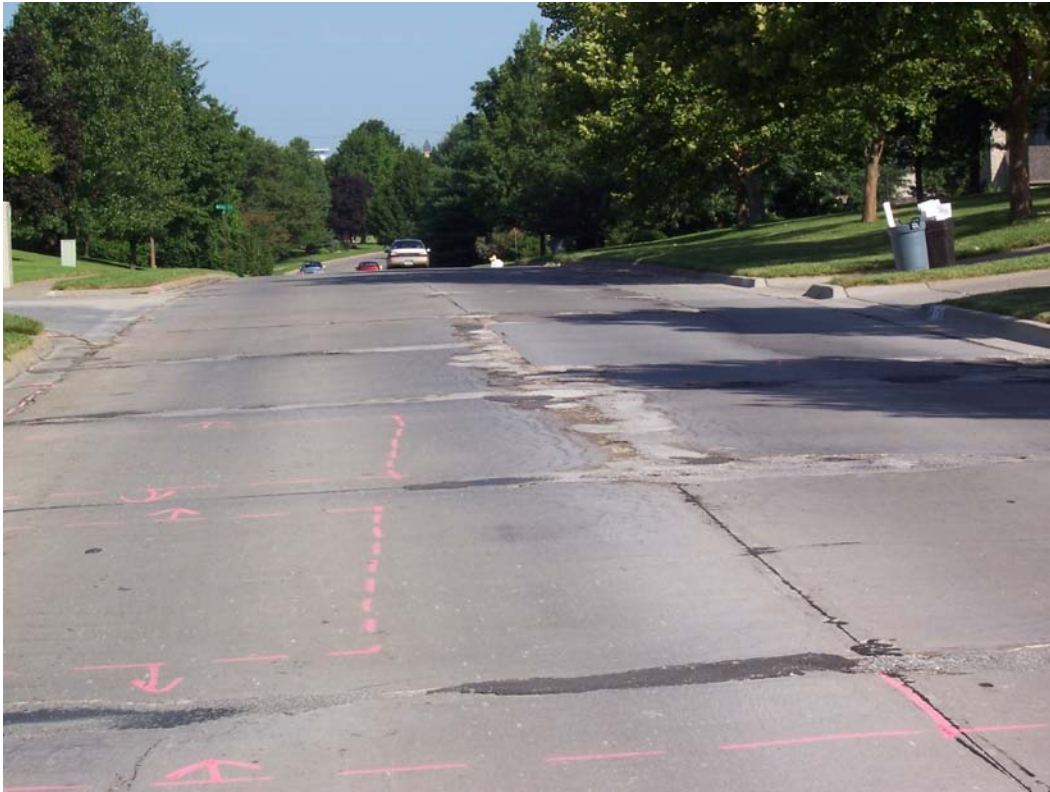
Description – Condition of Inverness Dr from Bob Billings Pkwy to Clinton Pkwy prior to Contracted Concrete Rehabilitation
