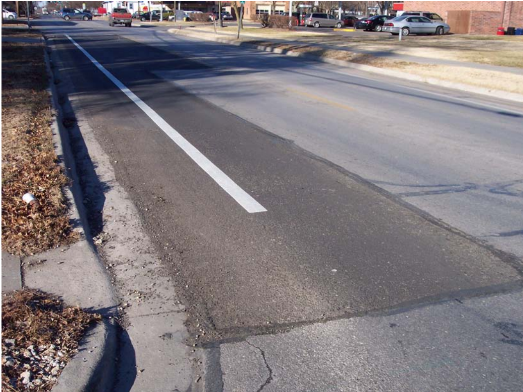
Description - Contracted Milling and Overlay Patching on E 19 th St from Massachusetts St to Barker Ave as part of Additional Area Patching
