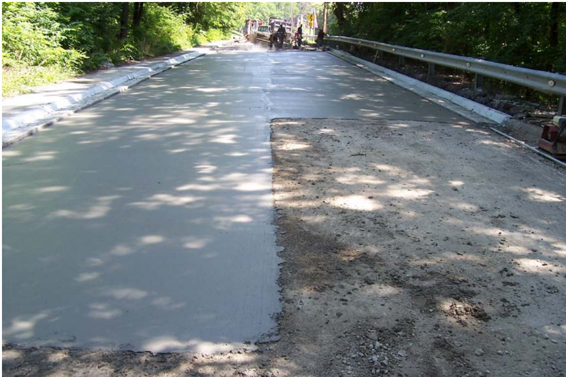
Description – Concrete base repair patching on Emery Rd from 9 th St to High Dr as part of Contracted Milling & Overlay (Phase 1 “Add”)
