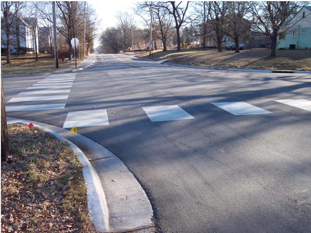
Description – Completed Overlay & Curb & Gutter Removal & Replacement on E 15 th St from Connecticut St to Haskell Ave as part of Contracted Milling & Overlay (Phase 2)
