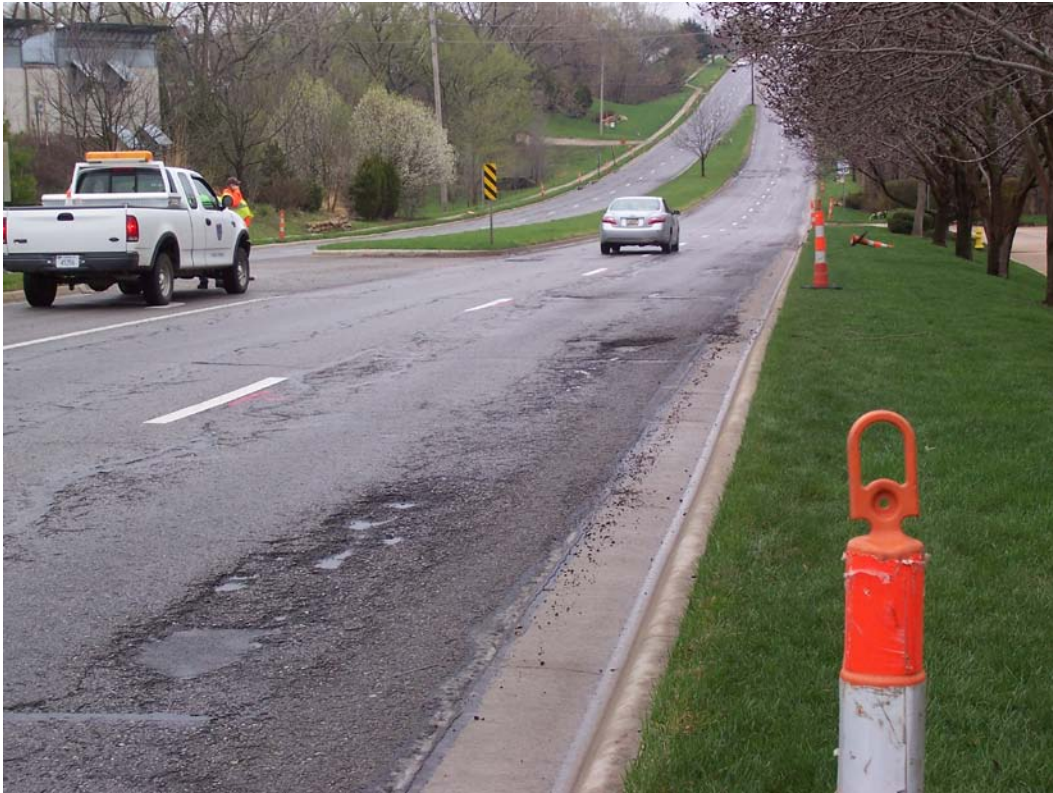
Description – Condition of Bob Billings Parkway near Wagon Wheel Rd prior to Contracted Milling and Overlay Patching as part of Emergency Repair and Rehabilitation
