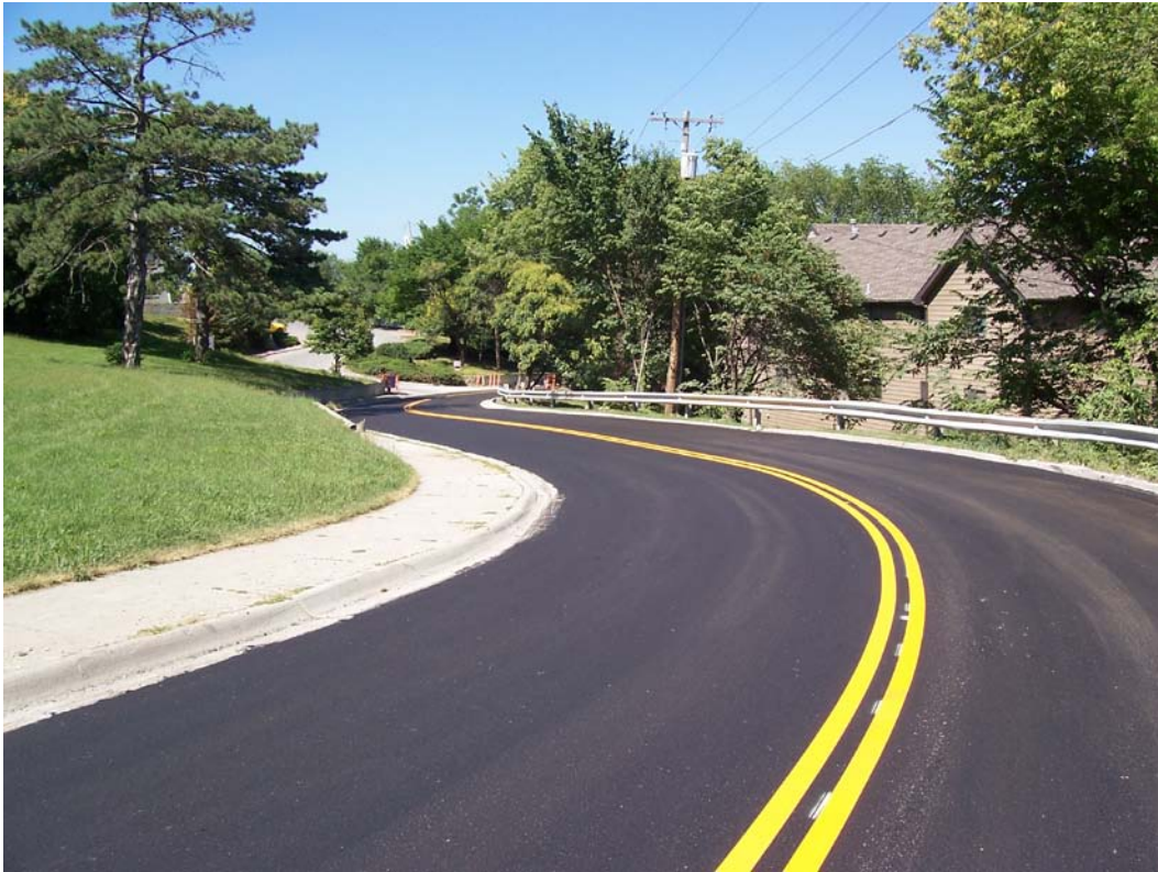
Description – Completed Overlay & Pavement Markings on Emery Rd from 9 th St to High Dr as part of Contracted Milling & Overlay (Phase 1 "Add")
