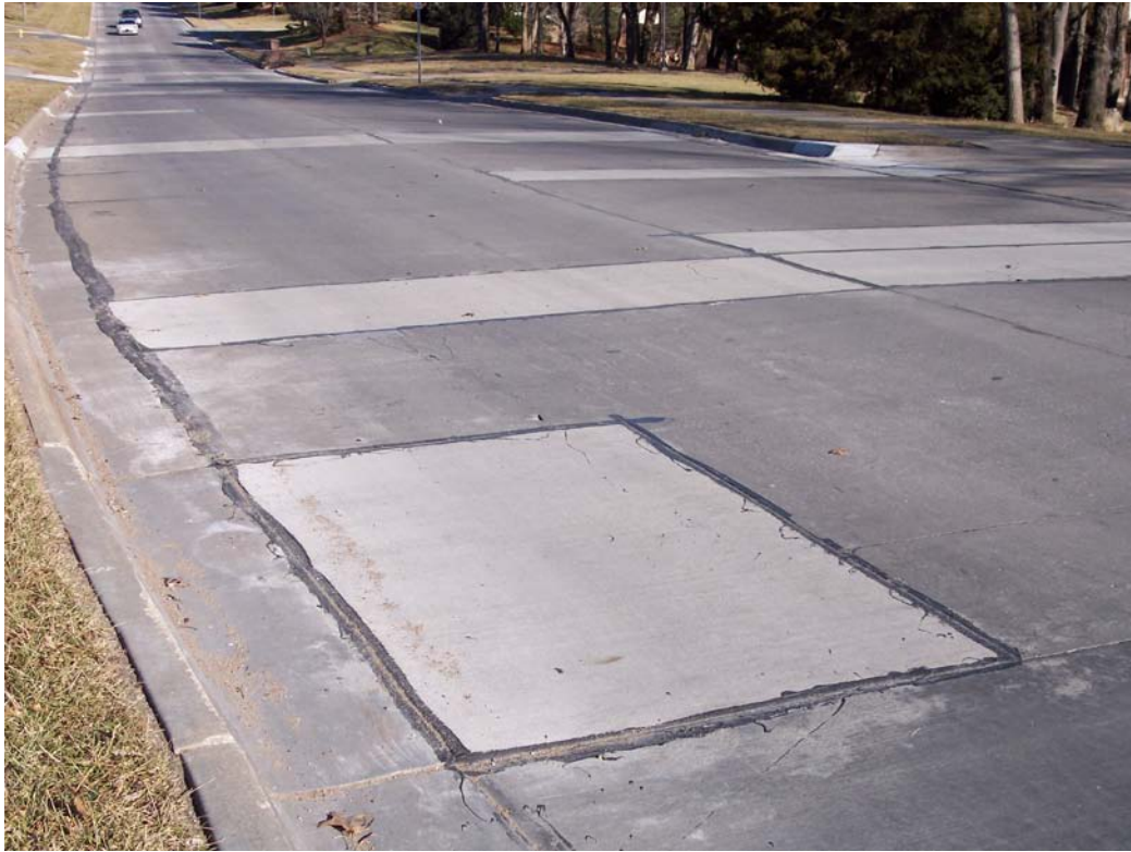
Description – Completed Concrete Patching w/ Curb & Gutter Repair on Inverness Dr from Bob Billings Pkwy to Clinton Pkwy as part of Contracted Concrete Rehabilitation
