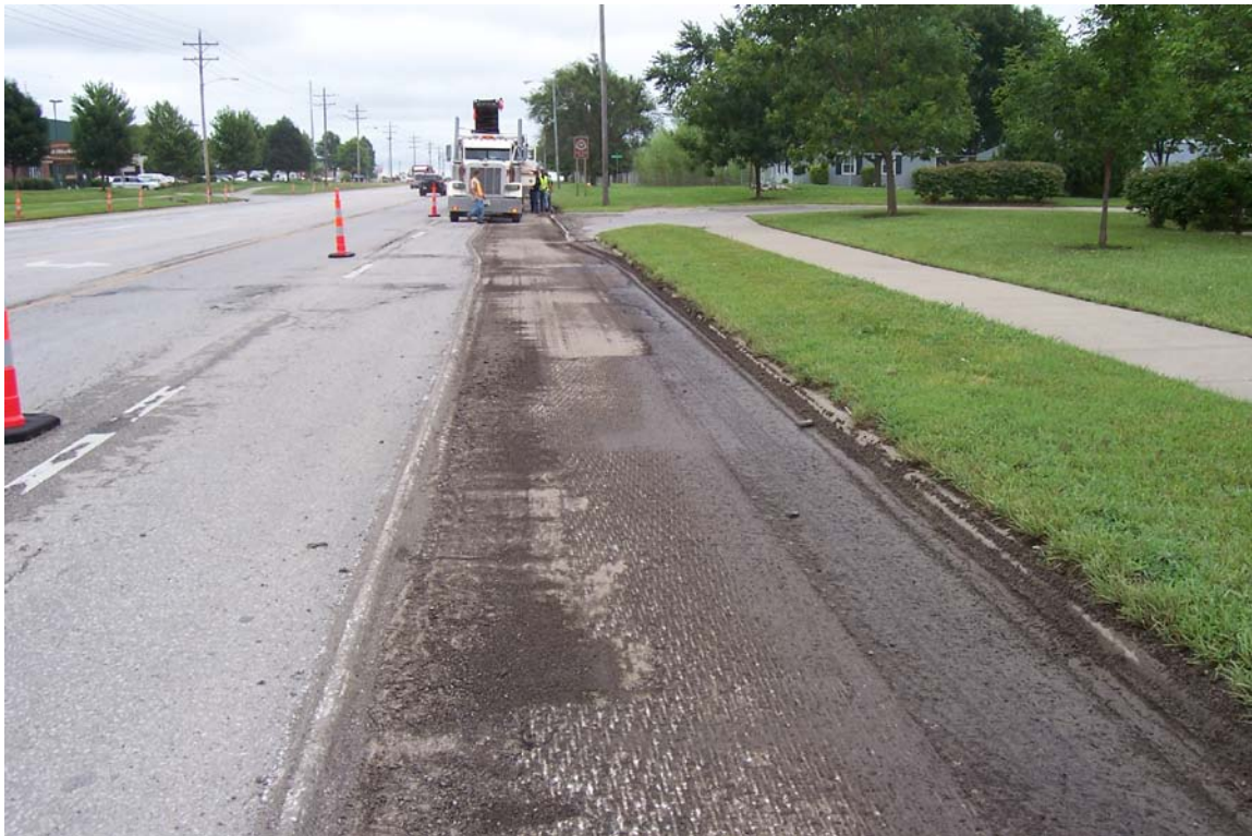
Description – Condition of E 23 rd St east of Harper Ave during Milling as part of E23rd St KLINK Milling and Overlay Project
