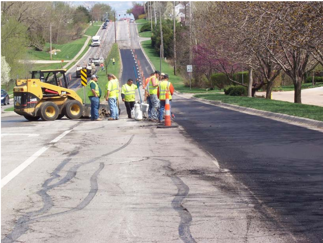
Description – Bob Billings Parkway near Wagon Wheel Rd after Contracted Milling and Overlay Patching as part of Emergency Repair and Rehabilitation
