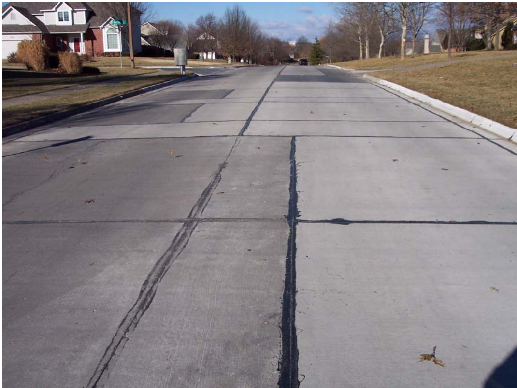
Description – Completed Concrete Patching w/ Curb & Gutter Repair on Inverness Dr from Bob Billings Pkwy to Clinton Pkwy as part of Contracted Concrete Rehabilitation
