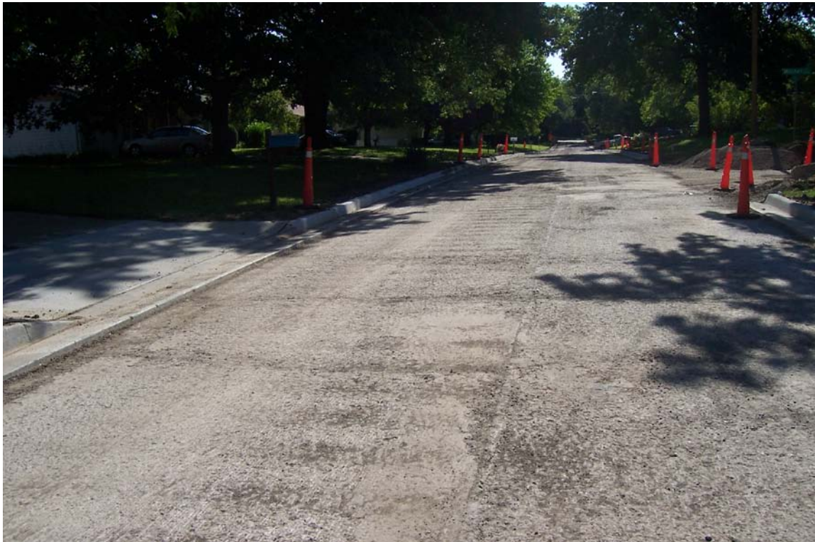
Description – Milled portion of W 20 th St near Mitchell St after Curb & Gutter Removal & Replacement as part of Contracted Milling & Overlay (Phase 2)
