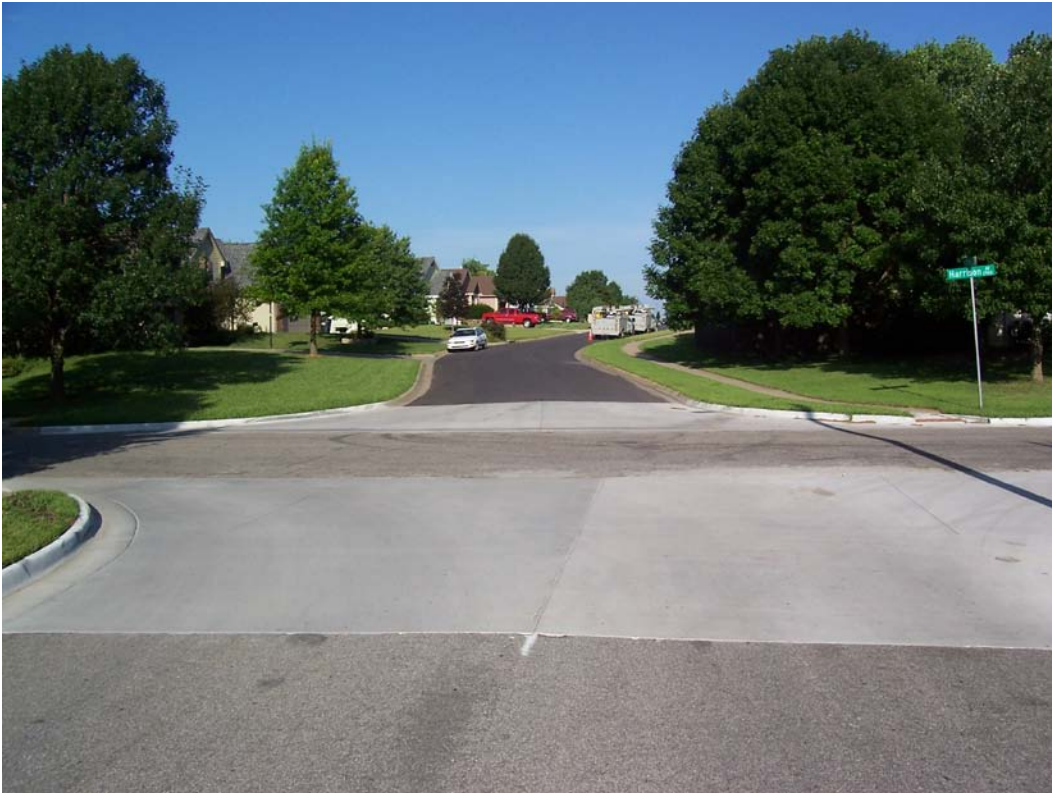
Description – Contracted Milling & Overlay (Phase 1) on 30 th St at Harrison Ave w/ coordinated concrete intersection work performed by Internal Street Division
