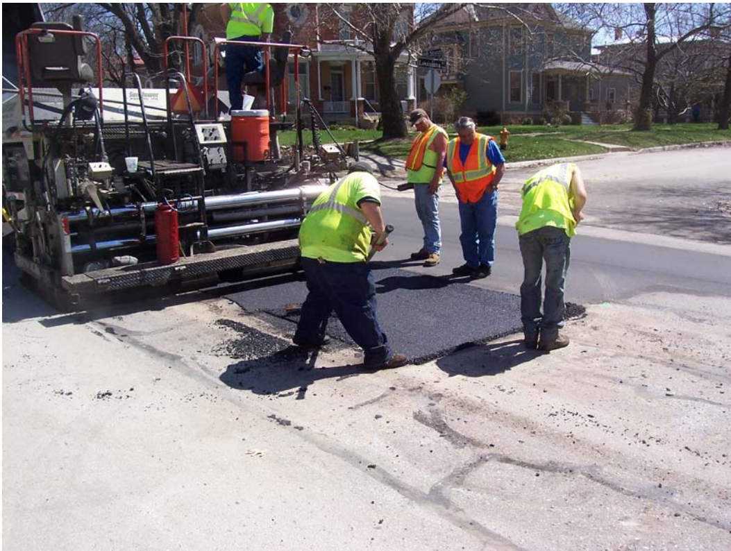
Description - Contracted Milling and Overlay Patching on W 6 th St as part of Emergency Repair and Rehabilitation
