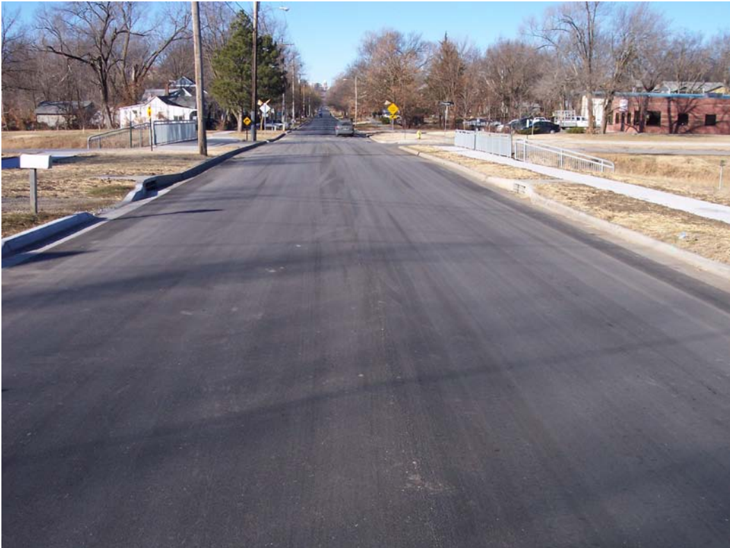
Description – Completed Overlay & Curb & Gutter Removal & Replacement on E 13 th St from Connecticut St to Haskell Ave as part of Contracted Milling & Overlay (Phase 2)
