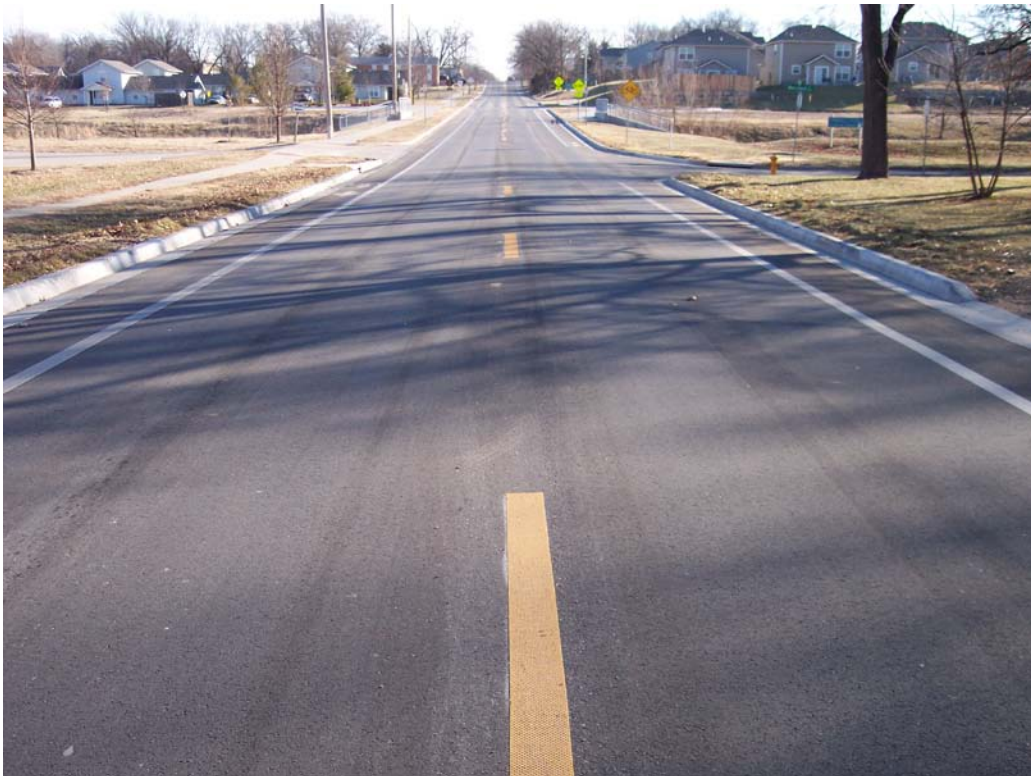
Description – Completed Overlay, Curb & Gutter Removal & Replacement, & w/ Bicycle Lane Pavement Markings on E 15 th St from Connecticut St to Haskell Ave as part of Contracted Milling & Overlay (Phase 2)
