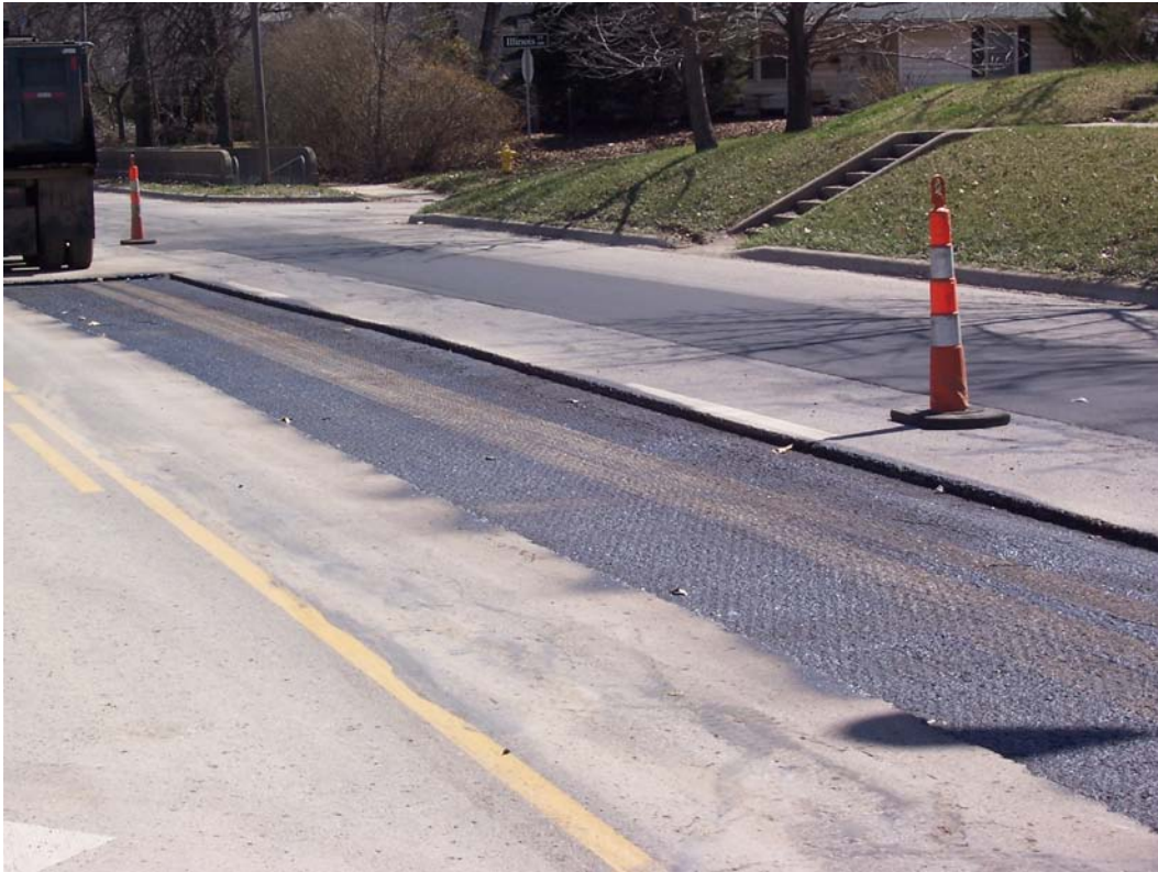
Description - Contracted Milling and Overlay Patching on W 6 th St as part of Emergency Repair and Rehabilitation
