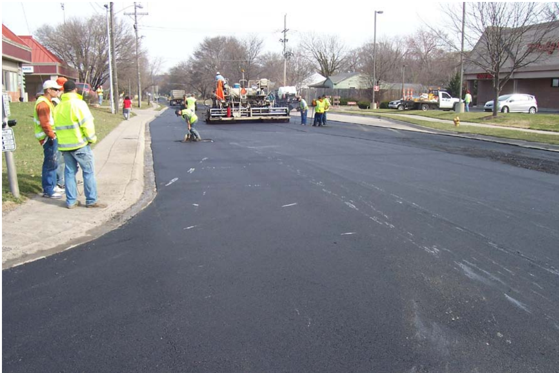
Description – Louisiana St near 23 rd St during Contracted Milling and Overlay Patching as part of Emergency Repair and Rehabilitation
