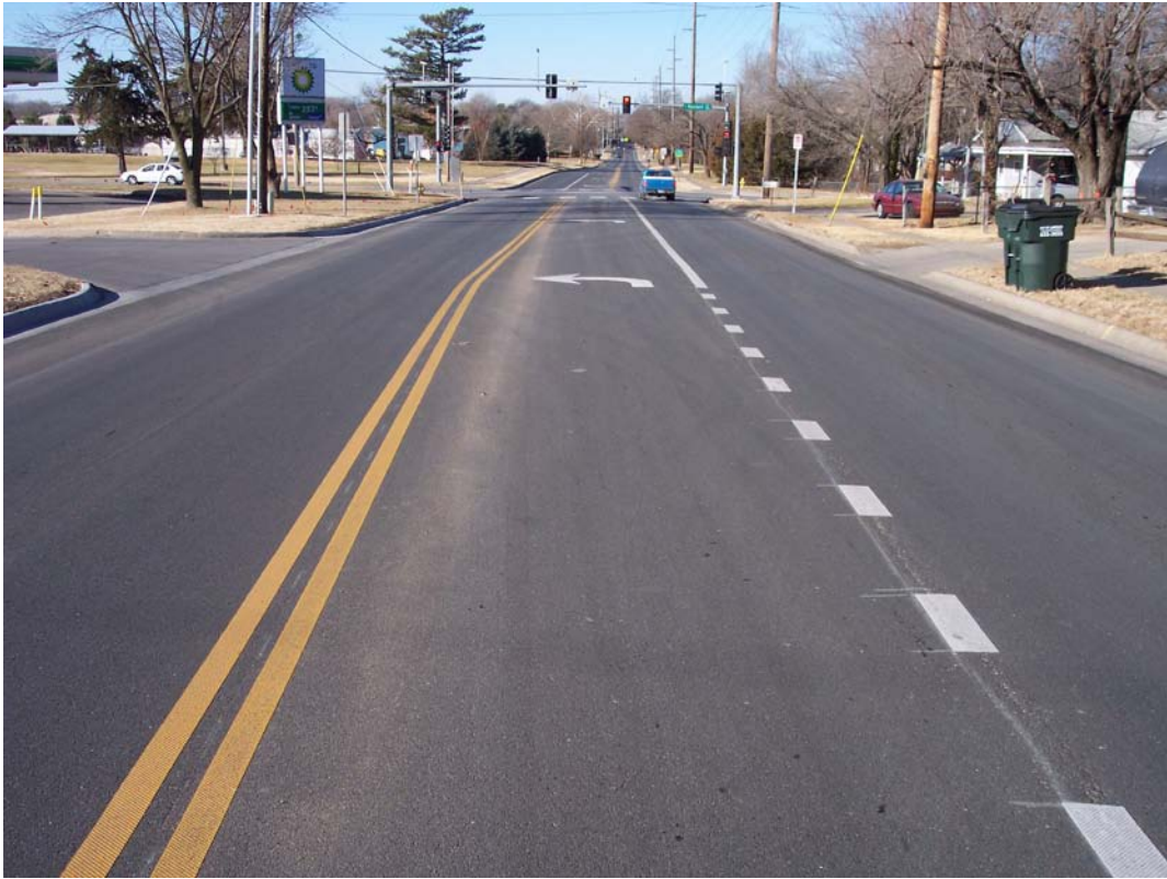
Description - Contracted Milling and Overlay w/ Pavement Markings & Bicycle Lanes on E 19 th St from Barker Ave to Almira Ave (E of Haskell Ave) as part of Emergency Rehabilitation
