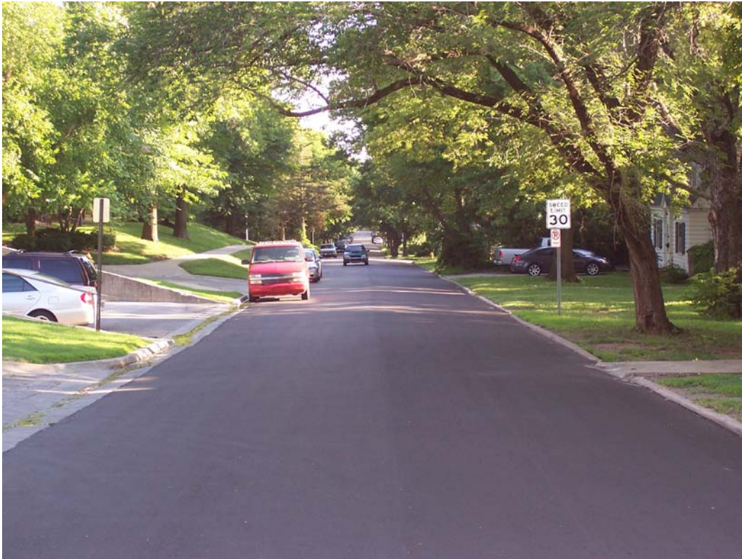
Description – Contracted Milling & Overlay (Phase 1 “Add”) on Missouri St near 11 th St
