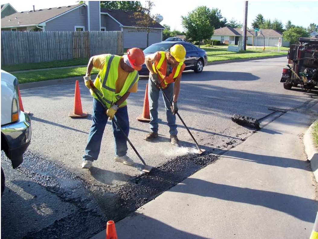
Description – Contracted Crack & Joint Filling w/ "PolyPatch" on Monterey Way N of W 6 th
