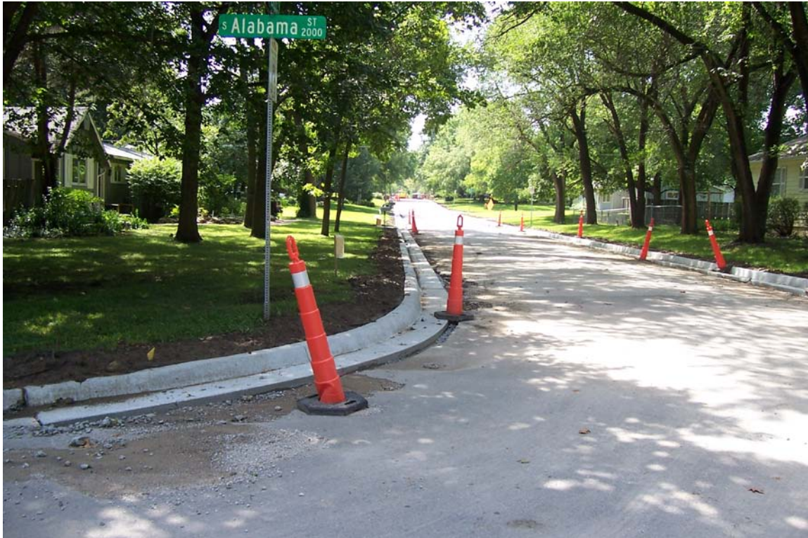
Description – Curb & Gutter Removal & Replacement on 20 th St west of Alabama St as part of Contracted Milling & Overlay (Phase 2)
