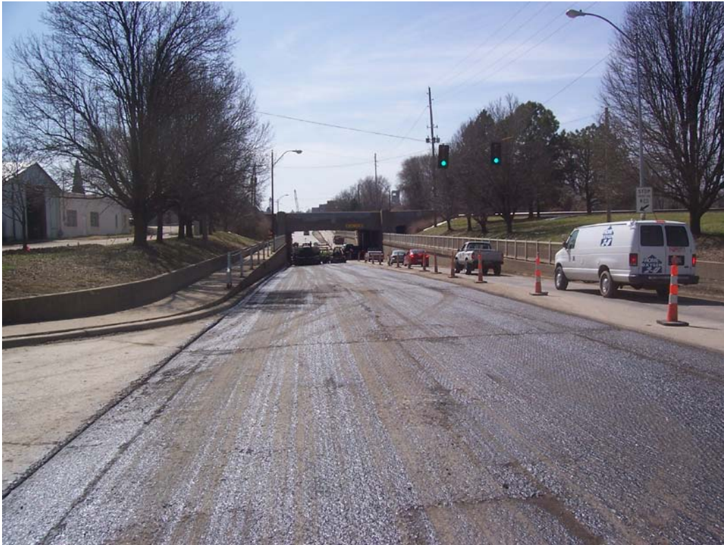
Description – N 2 nd St @ Lincoln St after Milling and just prior to Contracted Overlay as part of Emergency Repair and Rehabilitation in coordination w/ 2 nd & Locust Project
