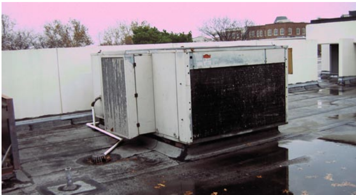
The existing 1972 Rooftop Units that need to be replaced for efficiency and condition.
