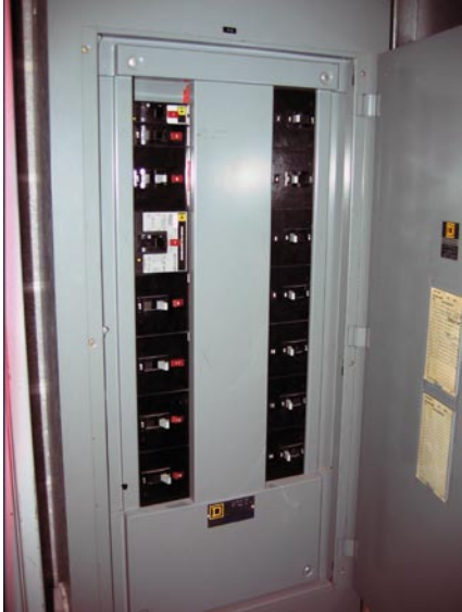
Existing main distribution panel board.
